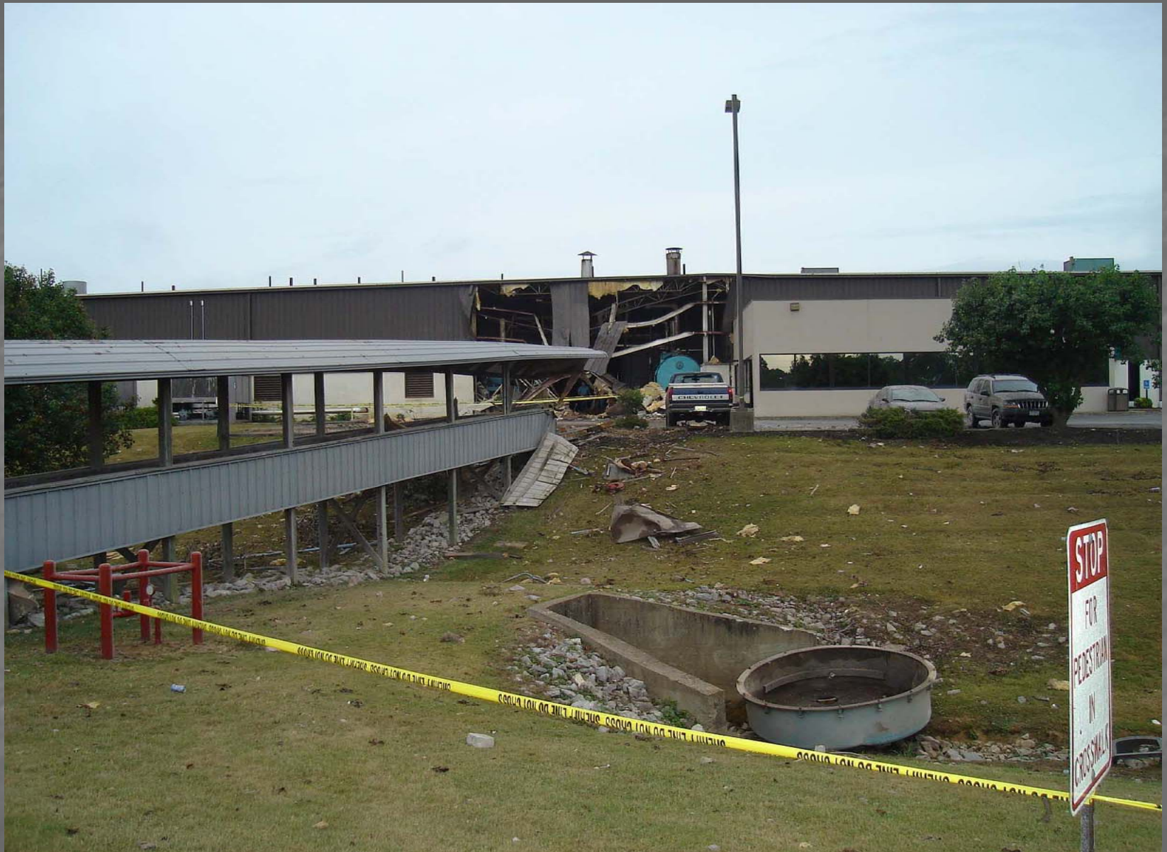
View of East Wall from Outside Plant (Note Rear Boiler Door in Ditch)
